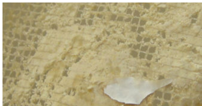
Removes inorganic scales
